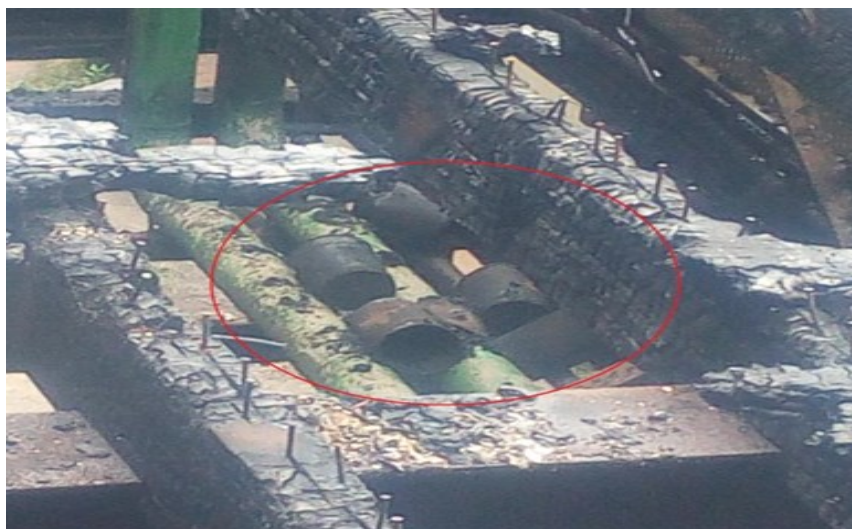
Cans believed to have contained flammable materials
